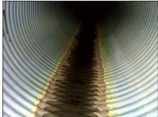
R1: Downstream view of the 407ETR culvert showing minimal standing water (Summer 2015).
