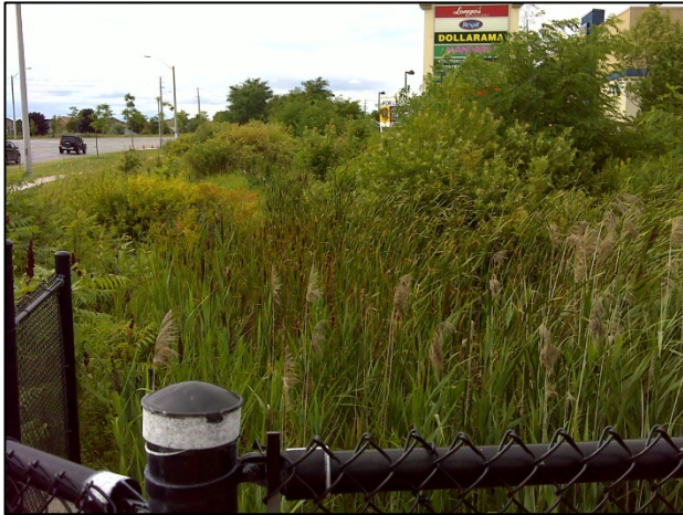
R5: Facing north (upstream) at structure inlet under Copper Creek Drive (Summer 2015).
